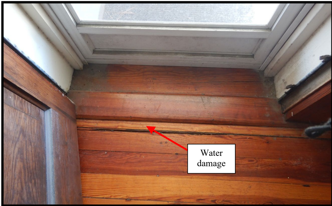
Photo #45 – Water damage at a sill plate.
