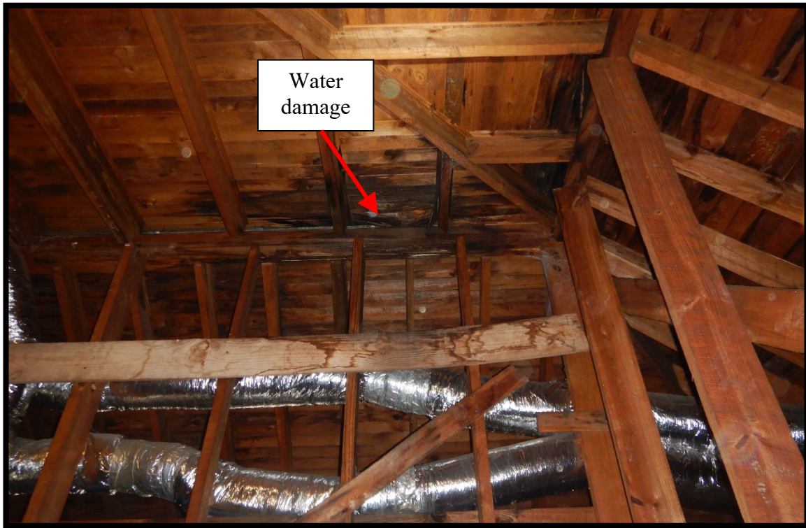
Photo #31 – Water damage under the top roof. It appears to be active.
