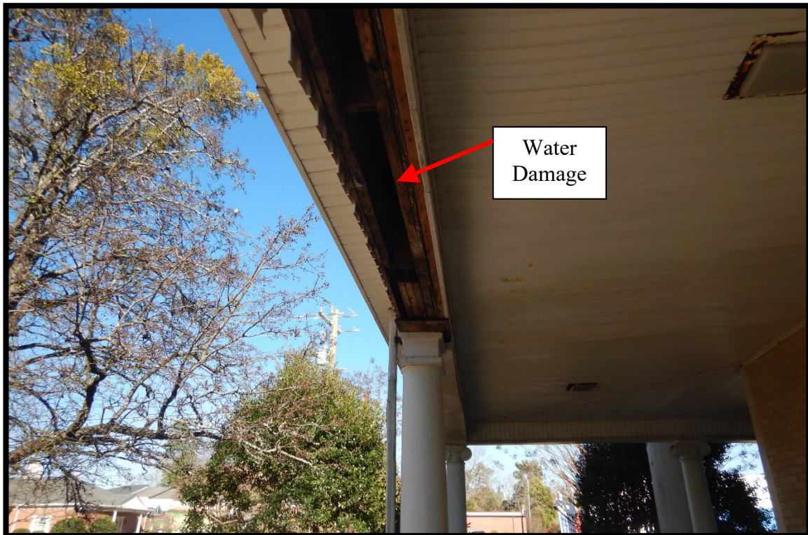
Photo #8 - This is the same water damage in photo 6.
