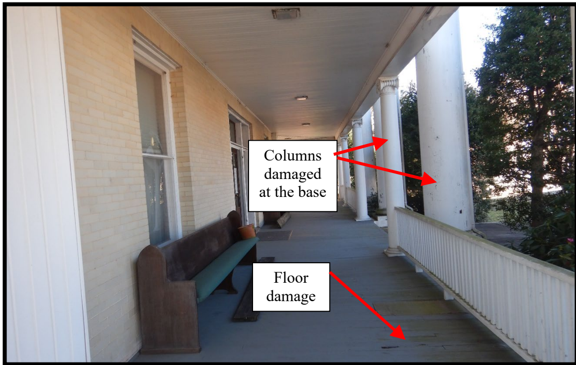
Photo #9 - This is a photo of the front porch. There is damage to the base of the large columns in front and damage to the tongue and groove deck.
