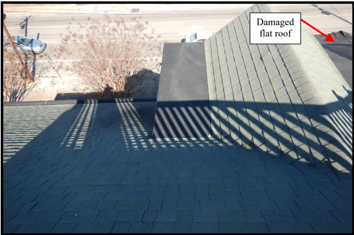
Photo #26 – There is damage to the front flat roof.
