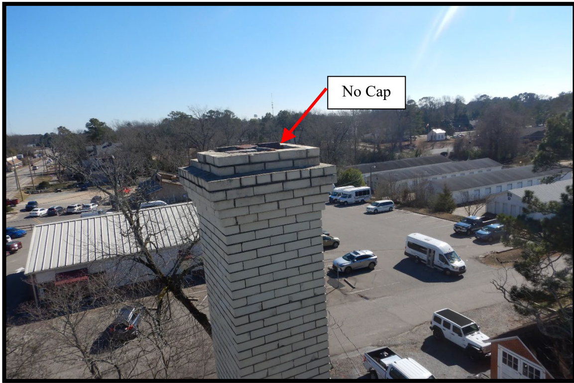
Photo #27 – There were no caps on the top chimneys.
