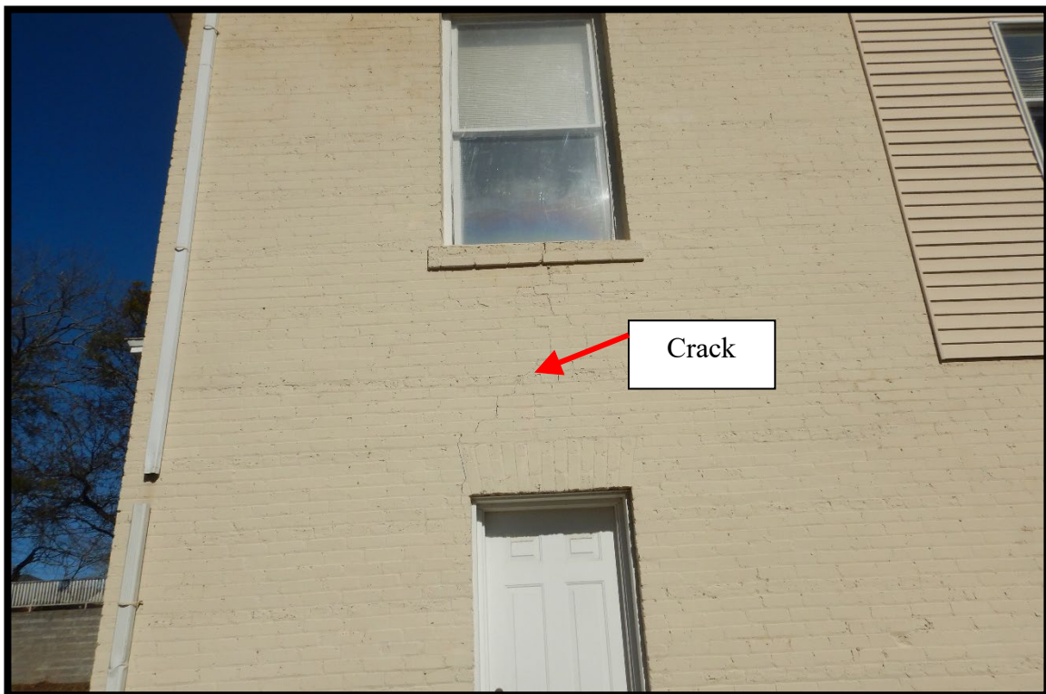
Photo #4 – Minor brick cracks at the rear elevation.
