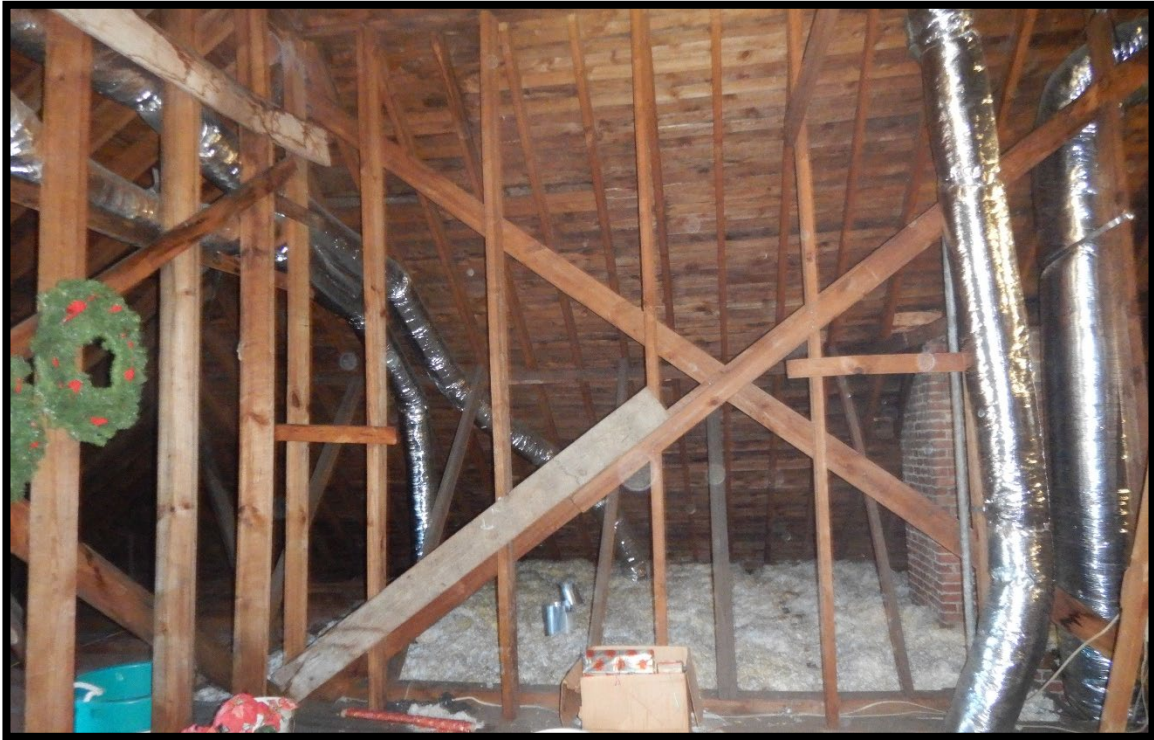
Photo #33 - This is a photo of the attic framing. The studs were all different sizes and spacings. Bracing was marginal.
