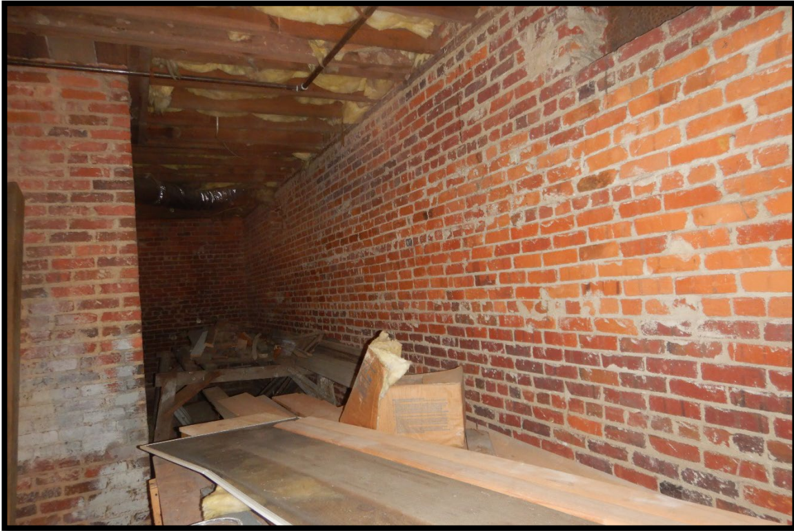
Photo #15 - This is the main structure basement foundation along the front. The walls are 12" thick solid brick.
