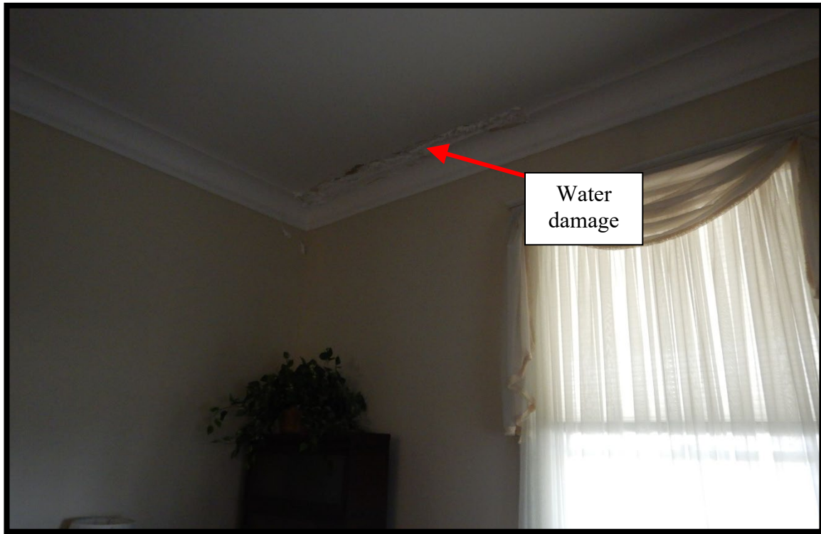
Photo #37 - This is a another photo of water damage.
