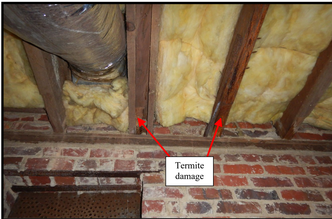
Photo #46 - This is a photo of termite damage in the basement.
