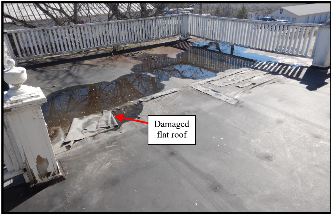
Photo #29 – Ponding water and damaged roof over the left porch cover in photo 10.
