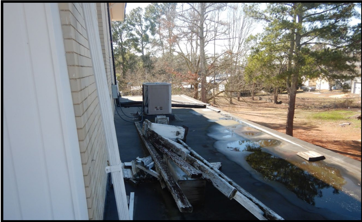
Photo #13 – This is the deck with the missing rail in photo 6. There is likely heavy hidden water damage.
