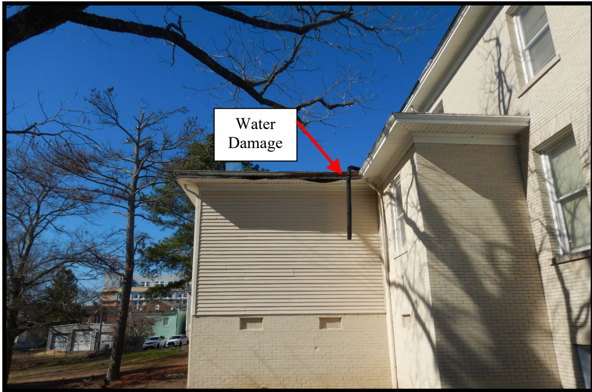
Photo #7- This is water damage at the rear left side.
