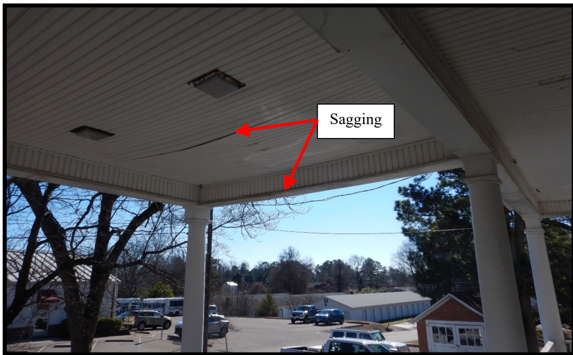
Photo #10 – The cover on the left side is sagging and there is likely heavy hidden water damage.
