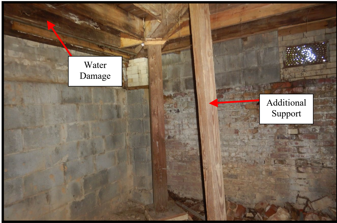
Photo #21 – Additional support added at the front left corner under water damage.
