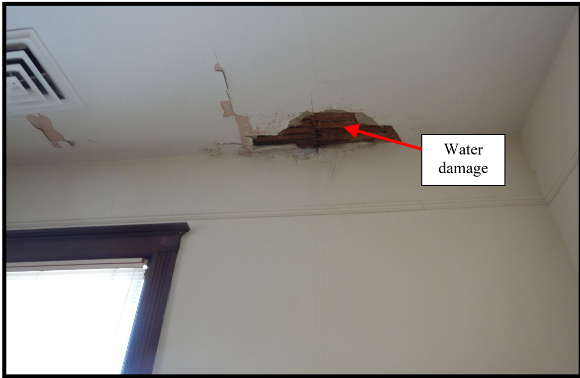
Photo #35 – Water damage in an upstairs room.
