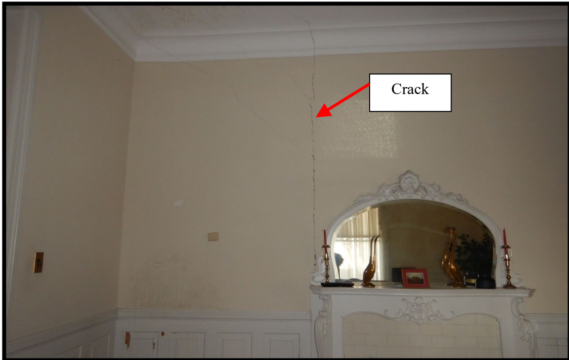
Photo #36 – Vertical crack in a downstairs room.
