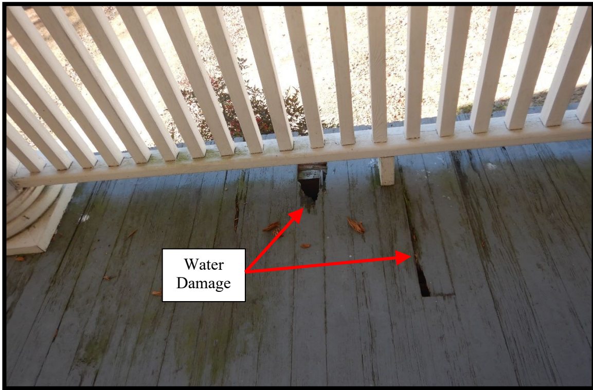
Photo #11 – Damage to the front porch decking.
