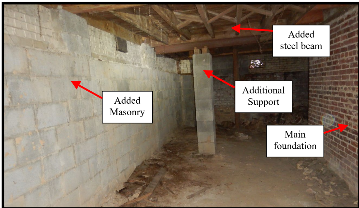
Photo #20 – Along the front porch wall additional block masonry was added to the brick. The owner stated that about 30 years ago there was a heavy rain that damaged the front wall, so it was reinforced.
