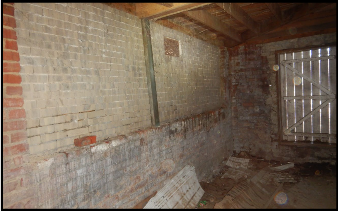
Photo #23 - This is the inside at photo 3. The brick is single wythe.
