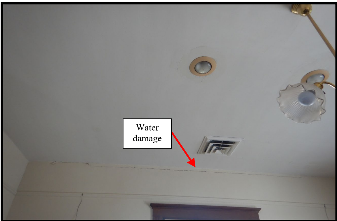
Photo #34 – Large crack in the stucco at the ceiling in an upstairs room.
