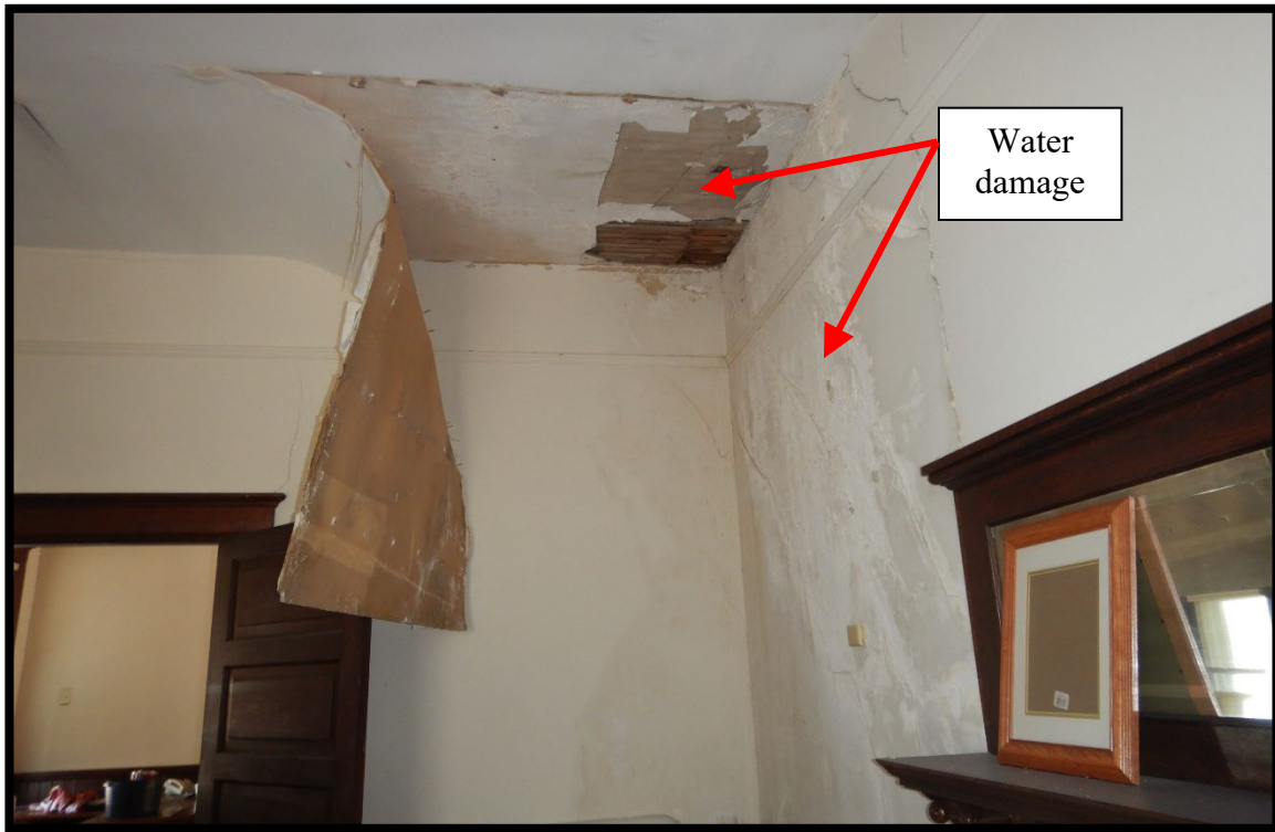
Photo #39 – Water damage downstairs, likely caused by a leaking HVAC pan.
