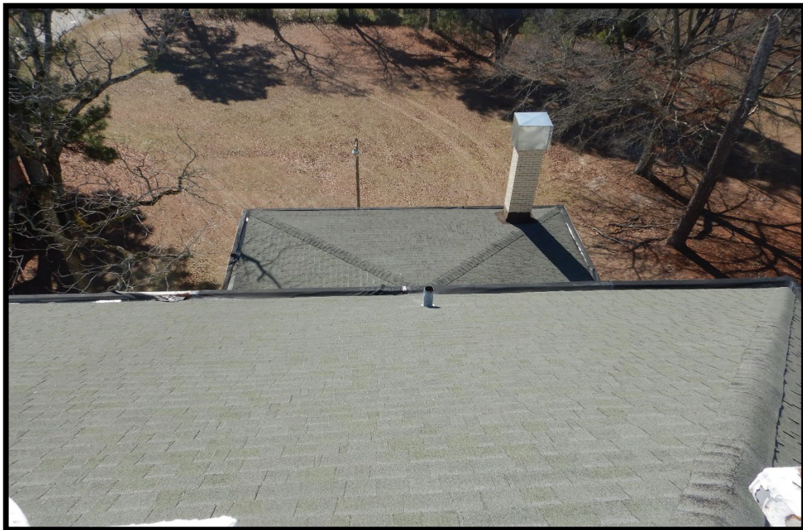
Photo #28 - There was a cap on the lower rear chimney.
