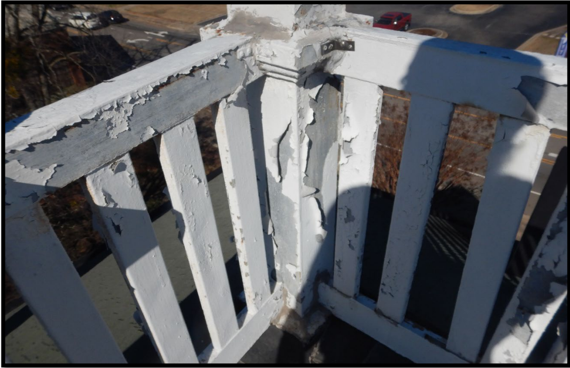
Photo #25 – Closeup of railing showing peeling paint.
