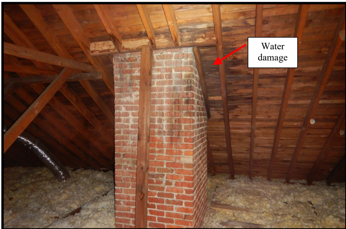
Photo #30 – Roof water damage around the left chimney.
