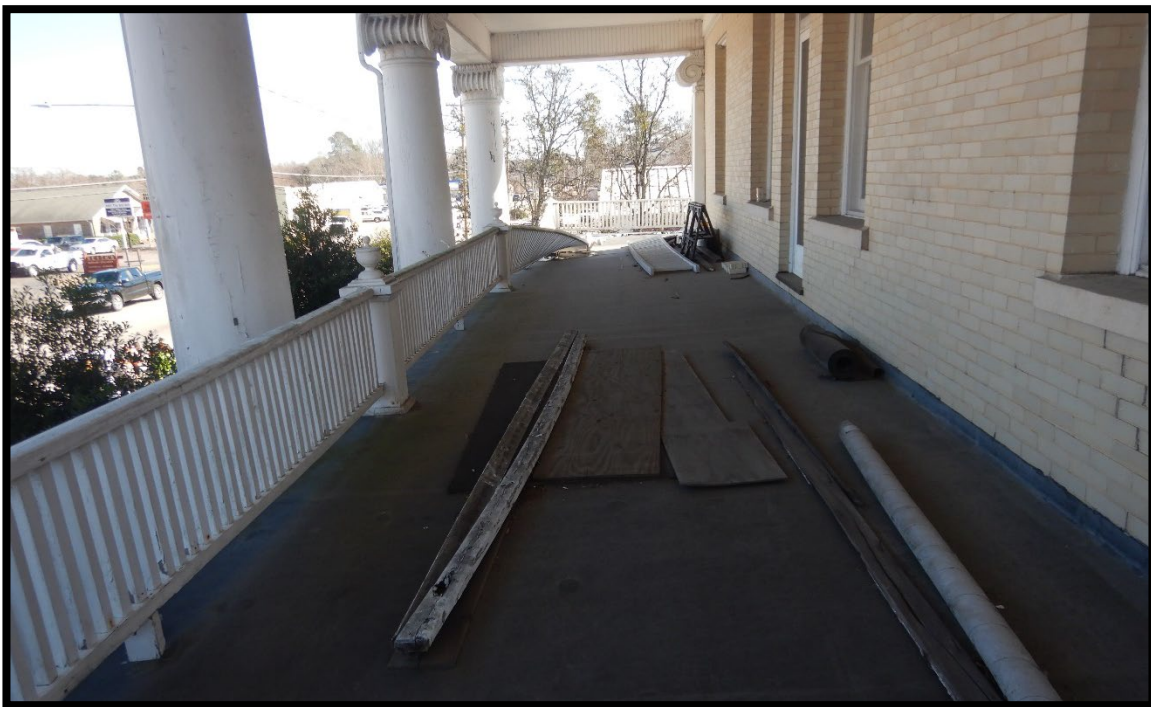
Photo #14 - This is the upper porch along the front. The porches were covered with an EPDM membrane roof approximately 40 years ago. There is likely heavy hidden water damage.
