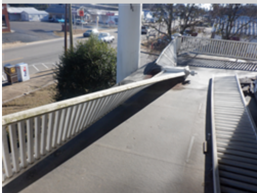
Image of damaged handrails on second story porch
