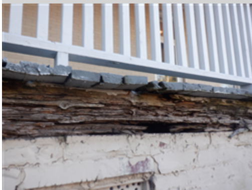
Image of decayed framing band and decking boards
